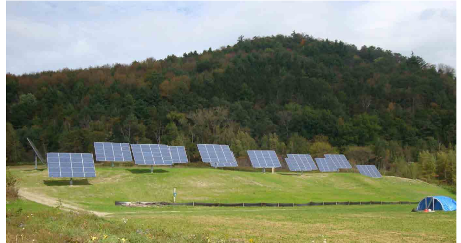
Solar photovoltaic installations along the edges of a farm field are an increasingly common sight.
