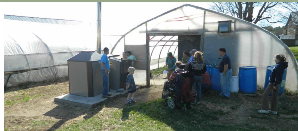
The Central Boiler Maxim 250 boiler installed at River Berry Farm in Fairfax, VT. These boilers may look like outdoor wood boilers common around Vermont, but they are EPA Phase II qualified due to improved emissions controls.
