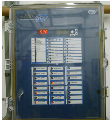
Ventilation controls provide optimal animal comfort and vary the air flow according to the conditions.
