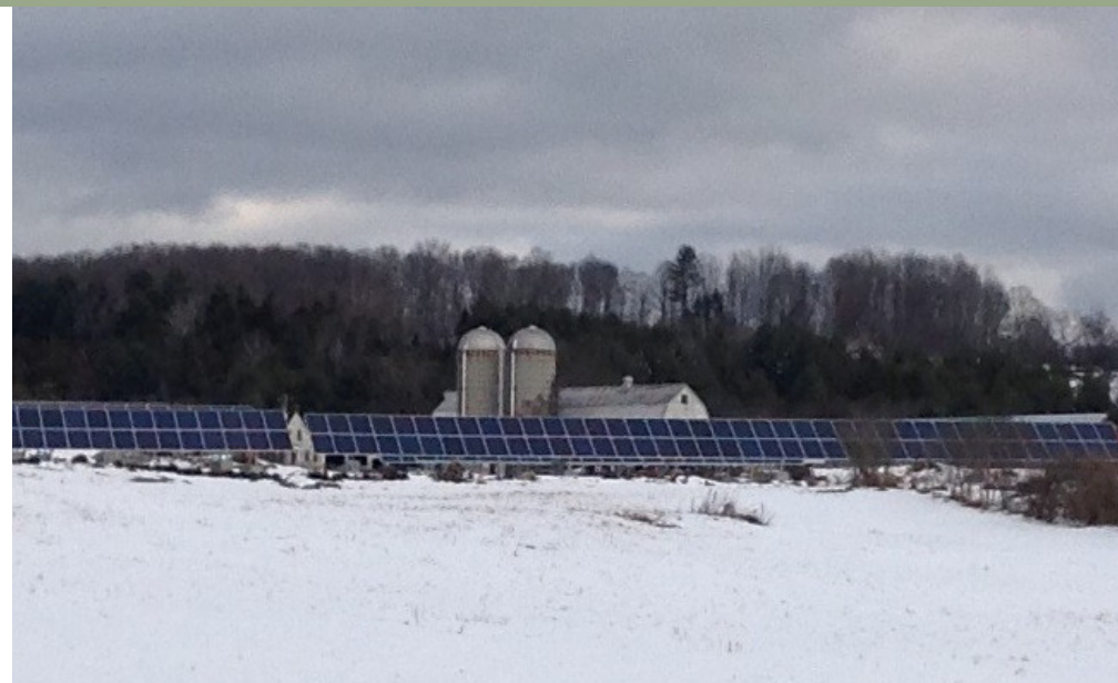
McKnight Farm solar array in East Montpelier, showing about one quarter of the 1.5-acre array, which is rated at approximately 95 kilowatts power output. The system was built by Catamount Solar.
