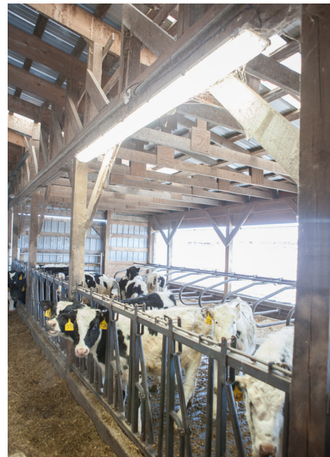
New vapor-proof lighting in the dry cow barn.
