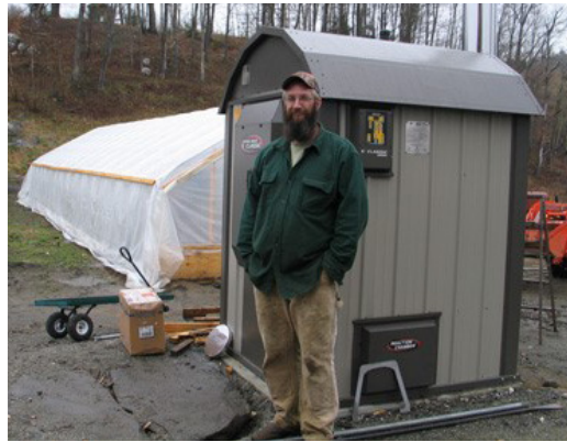
Paul Betz uses the Central Boiler eClassic to heat two greenhouses with cord wood.
