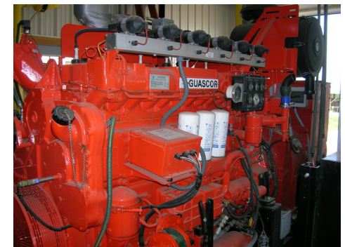
Guascor engines are commonly used with methane digesters in Vermont.
