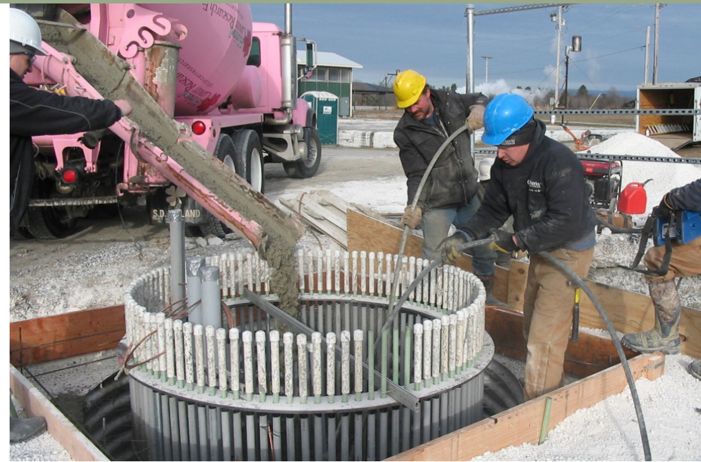
A below-ground pad of reinforced concrete is connected to a ring of rods (the "bolt cage"), visible in the photo, that rise to a few inches above ground level. This ring will also be encased in concrete, except for the top few inches, onto which the tower is bolted. Also shown are the electrical conduits, which will come up through the concrete floor inside the tower.
