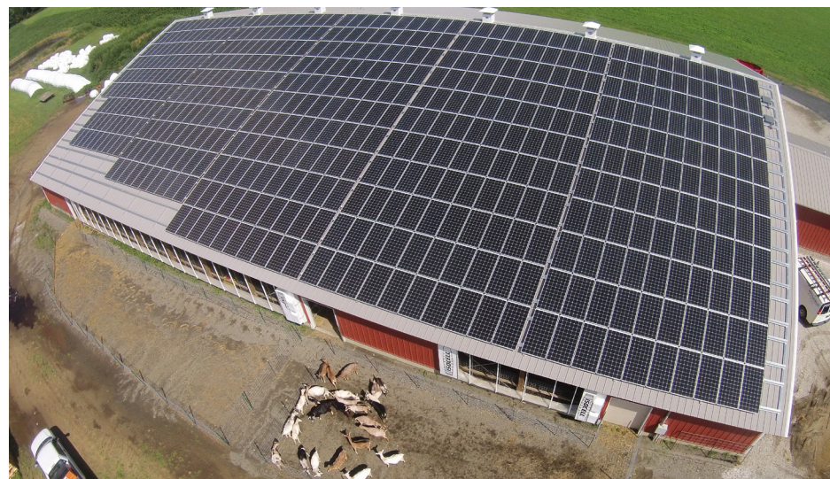
The 572 solar panels, here shown almost fully installed, use the one-third-acre south-facing roof, mounted on a frame designed by Aegis Renewable Energy. The image was captured using a remote-controlled helicopter.
